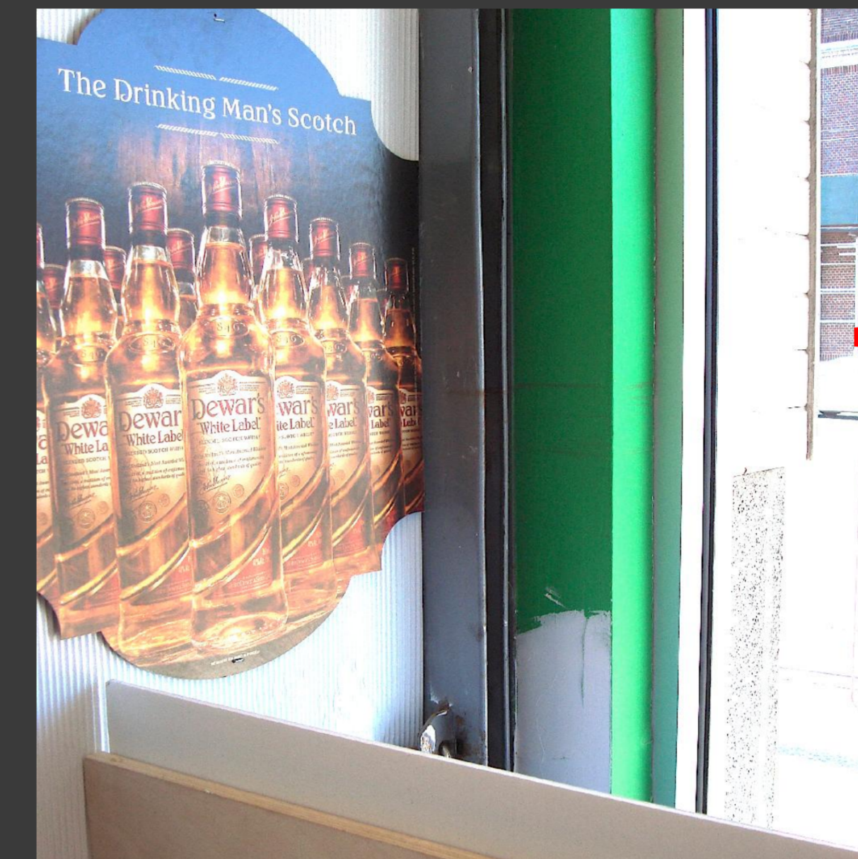
Signs of Flood Damage on the Beam in a Business © Helen Jankovski
